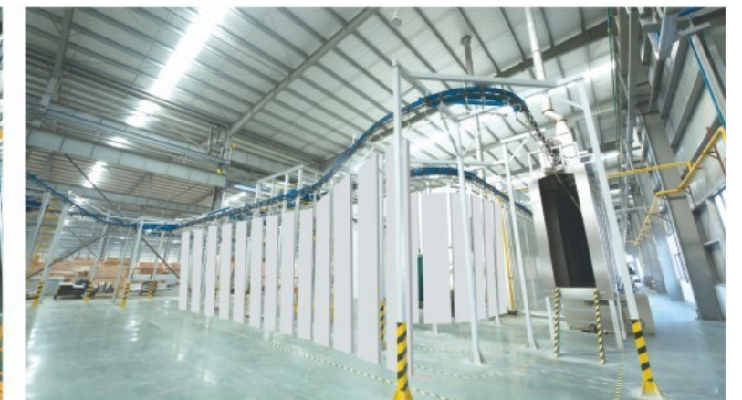
Spraying Line (German WAGNER Spraying Room)
